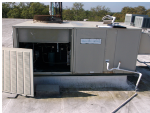
Existing Roof Top 100% Outside Air Unit
