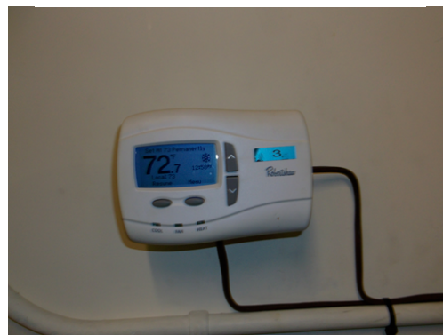
One of the existing thermostats
