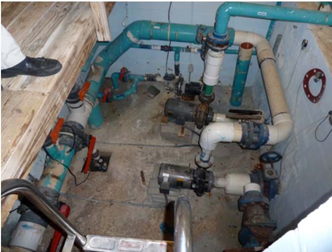
Existing Pool Pumps
