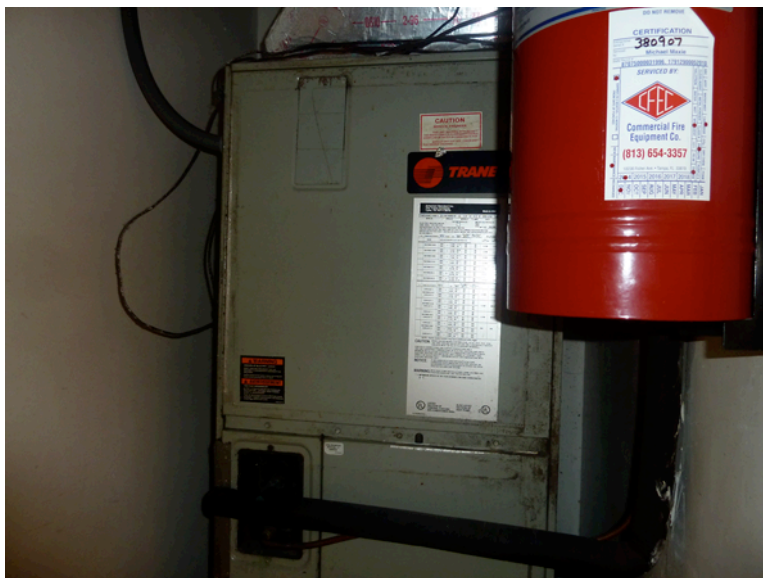
One of the systems to be replaced
