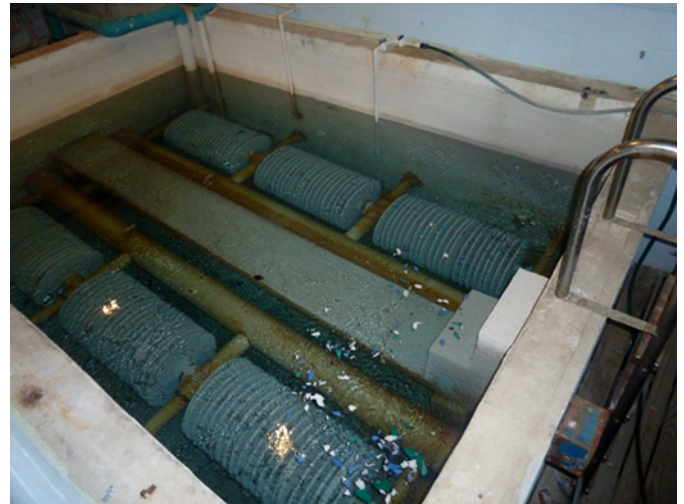
Existing DE Filtration System
