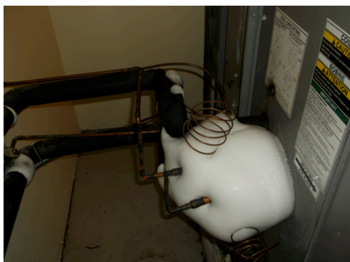
Some of the issues with the existing systems
